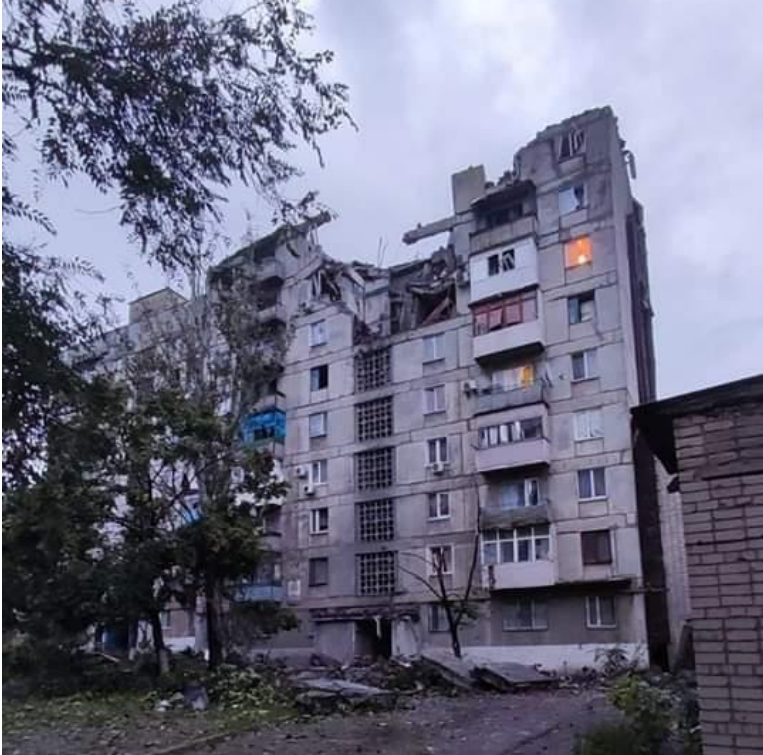
An apartment building hit by shelling in Alina's hometown of Toretok.
